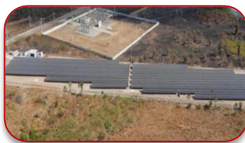
Amontada II ENEL - CE 1.2 MWp
