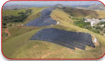
Angra Light - RJ 4.6 MWp
