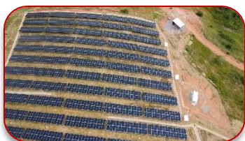
Carmo FE Light - RJ 5.3 MWp
