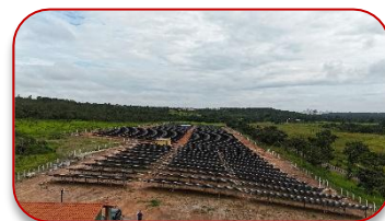
Catena Cemig - MG 3.6 MWp
