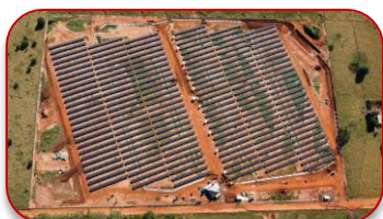
Santa Maria Energisa - MS 3.4 MWp
