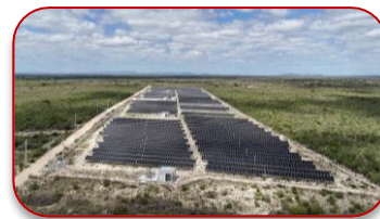
Petrolina Neoenergia - PE 5,0 MWp
