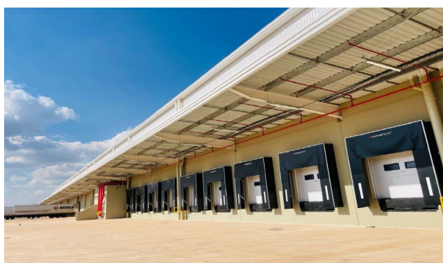
Docas com Dock-shelter Módulo 5 – BTS Libbs.
